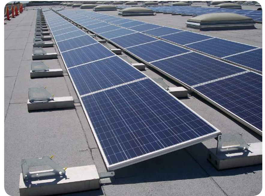
Precedent image of rooftop solar installations
